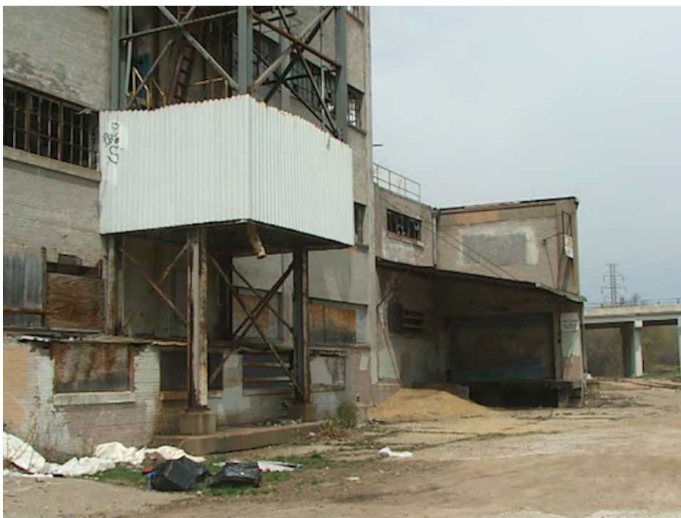
Photo 20: Deterioration and demolition of Fruen Mill.
