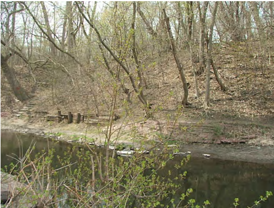
Photo 18: Bassett Creek Park Retaining Walls, staircase, and erosion.
