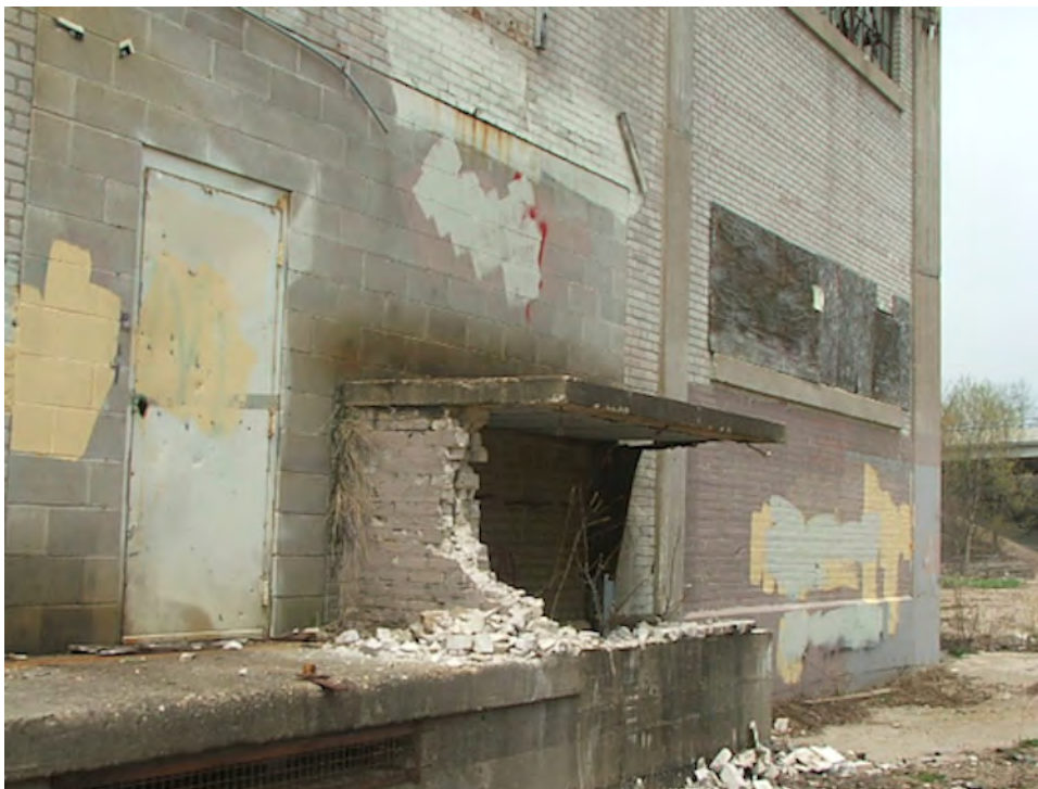
Photo 19: Deterioration and demolition of Fruen Mill.
