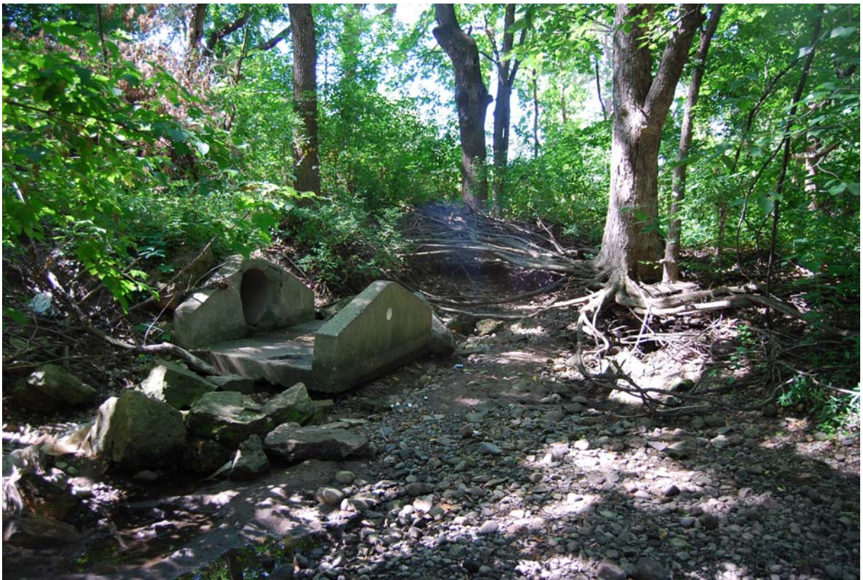
Stormsewer outlet and bank erosion at Site 14.
