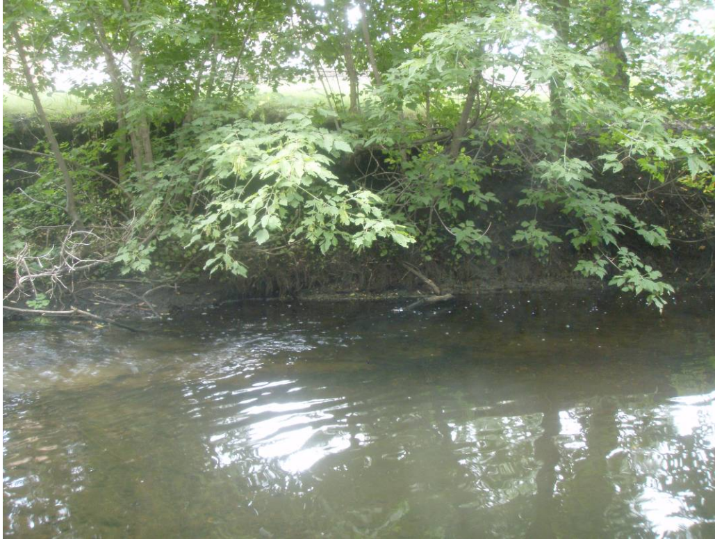
Photo 15. Site 15. Minor bank erosion.
