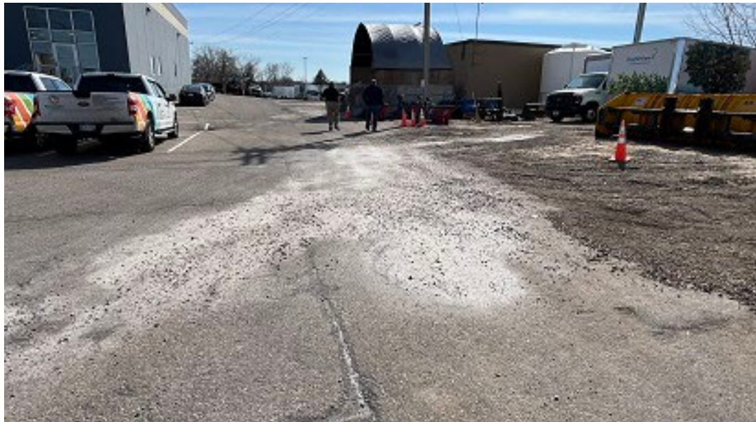
Salt residue on pavement near equipment storage area
