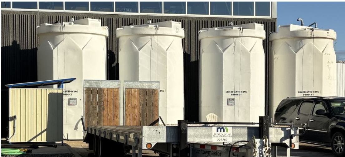
Liquid storage tanks and brine blending shed
