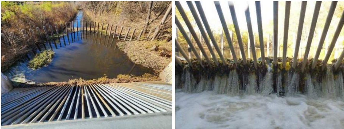
Figure 3-1 Trash Rack Debris Prior to Cleaning (Typical)
