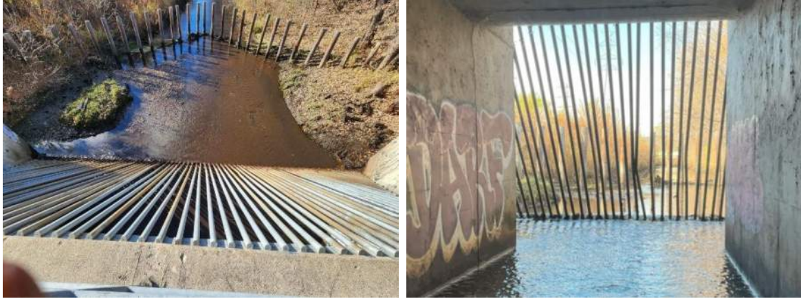
Figure 3-2 Trash Rack Debris Following Cleaning By City of Minneapolis
