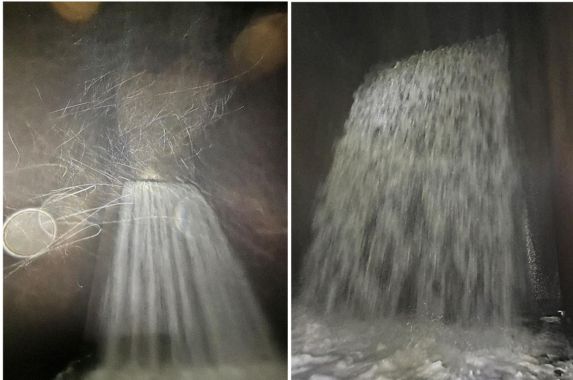
Figure 3: Drop Structure from Double Box Culvert to 3rd Ave. Tunnel (blurry due to heavy mist)
