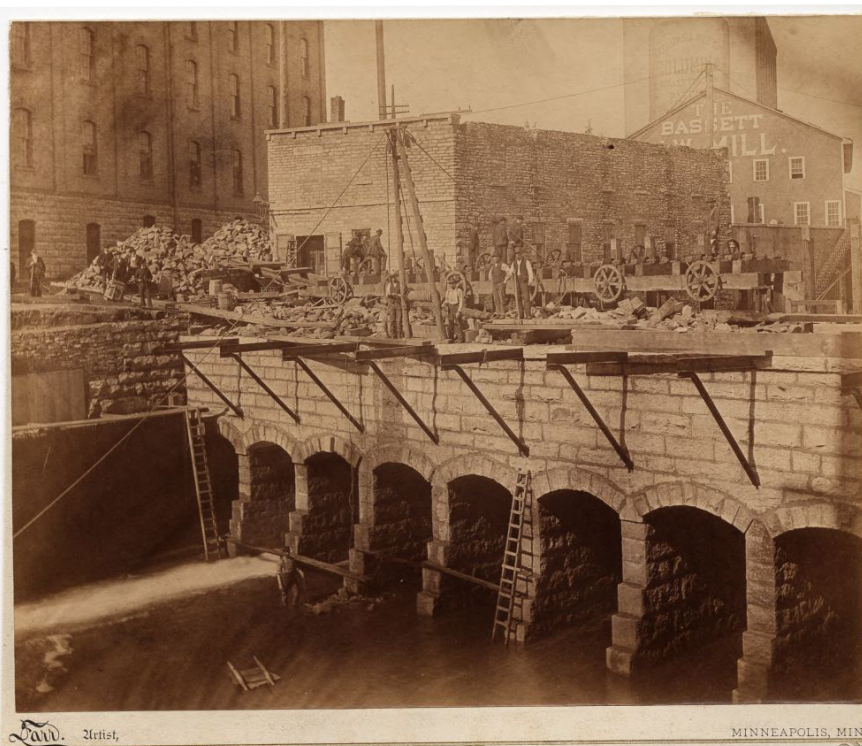
Construction of the main canal and gate house on the West Bank of Mississippi River, with Bassett Sawmill and Columbia Flour Mill in the background
