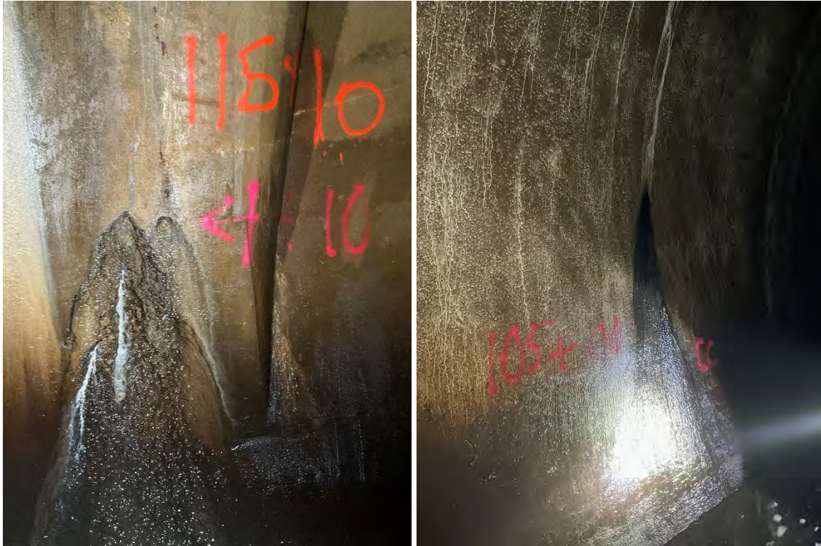
Figure 6: Example of an Infiltration Weeper (IW) (left photo) and an Infiltration Runner (IR) (right photo)
